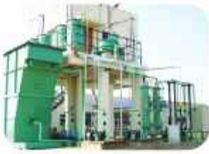
Effluent Treatment Plant
